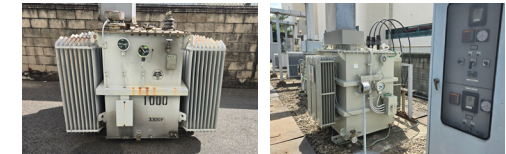
Before Replacement (Aging Transformer)
